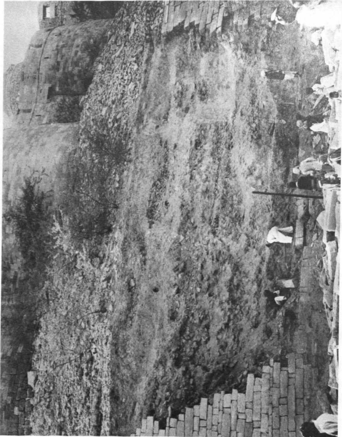
174 Jaisalmer Fort : Lower fortification wall near nichipole before conservation. See page 231
