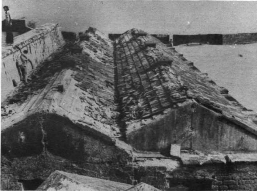
136. Fort St. Angelo, Cannanore : Showing the leaky terrace of the horse stables before conservation. See page 223
