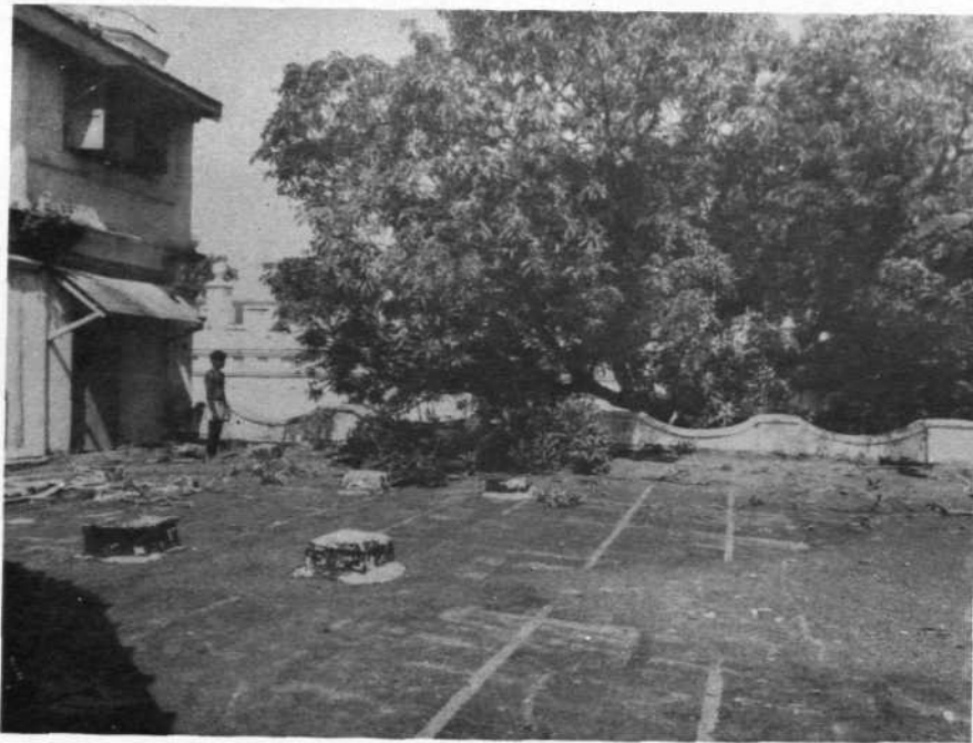
140 Big-ware house Fort St. George Madras : View of the decayed Madras terrace roof before conservation. See page 224
