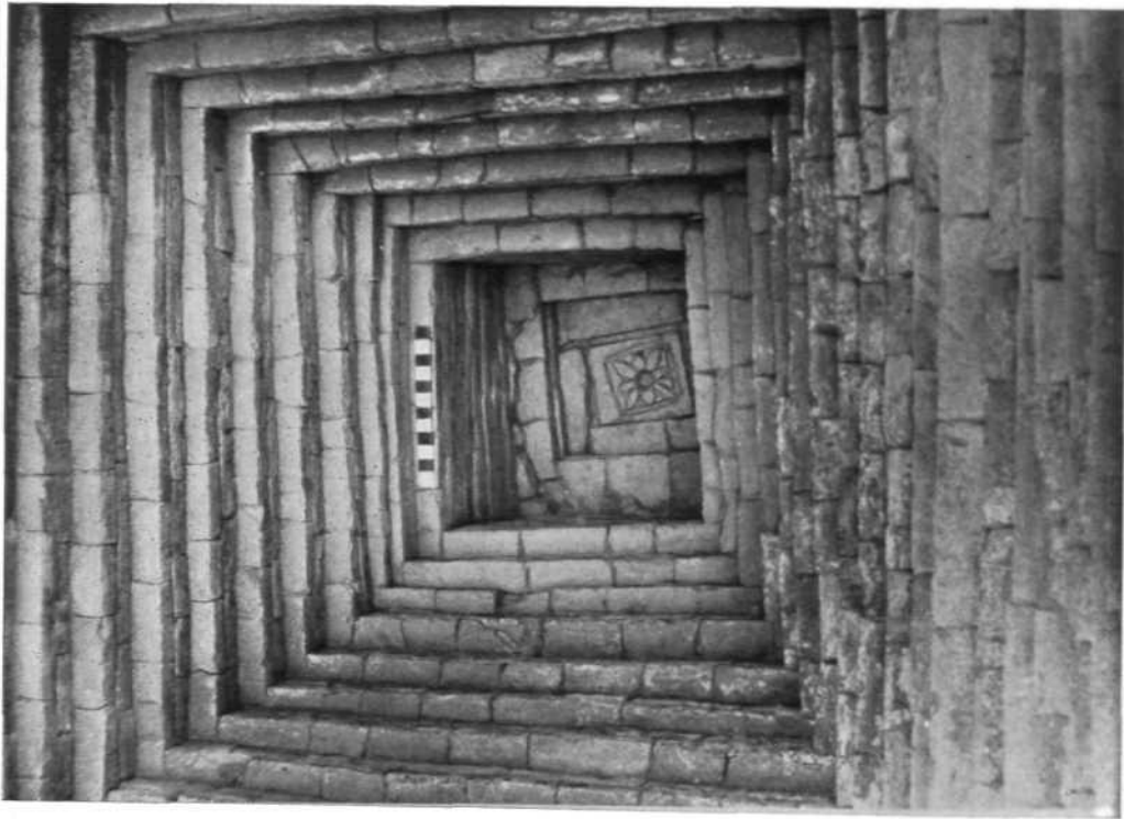
B Chandraketurah : A, Khana-Mihirer-Dhipi, main temple showing earliest working-levels; B, kunda with foundation-tablet carved with lotus. See p. 52
